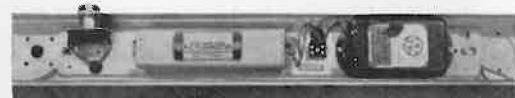
4 The interior of a present-day Mazda fluorescent fitting showing auxiliary gear mounted on a tray.
