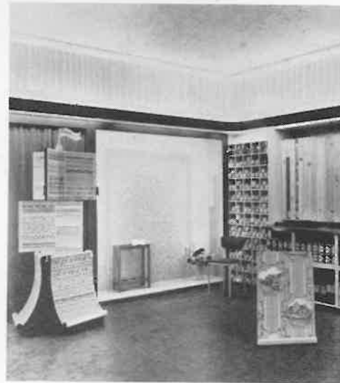
Cornice lighting with fluorescent lamps concealed by a wooden pelmet in the Wallpaper Stores Ltd. Oldham.
